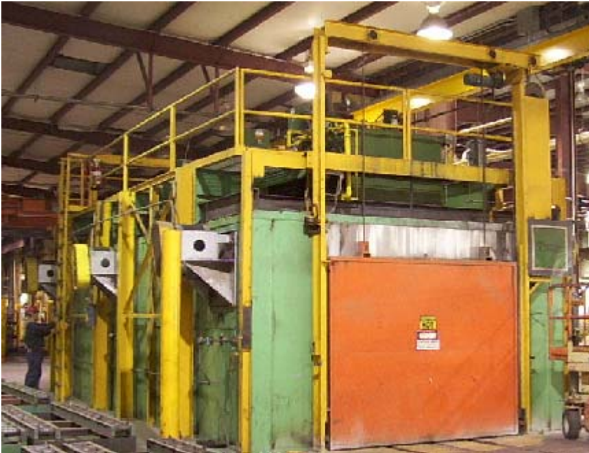
The oven before the six foot extension.
