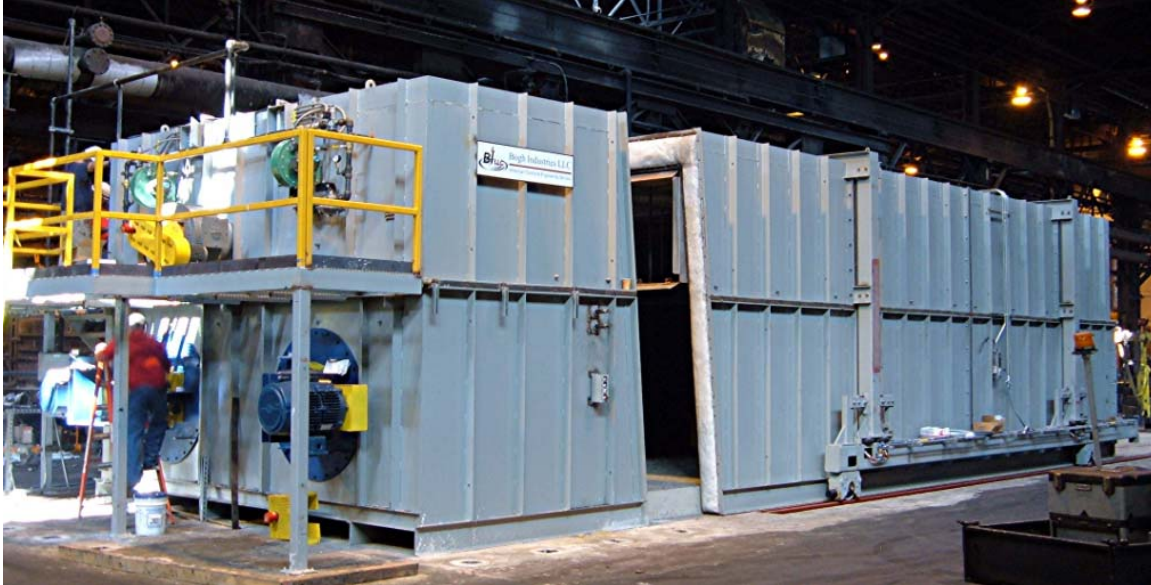
Figure #7. The picture shows the oven during final installation.
