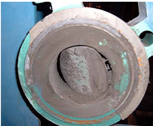
Figure #1 The picture shows an air control valve removed for inspection with a large buildup of dirt.
