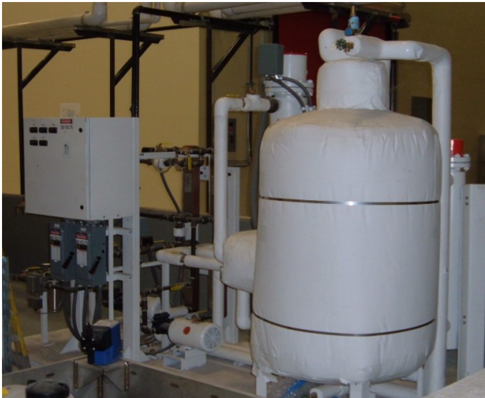
The picture shows the new heat separator installed at the customer site.
