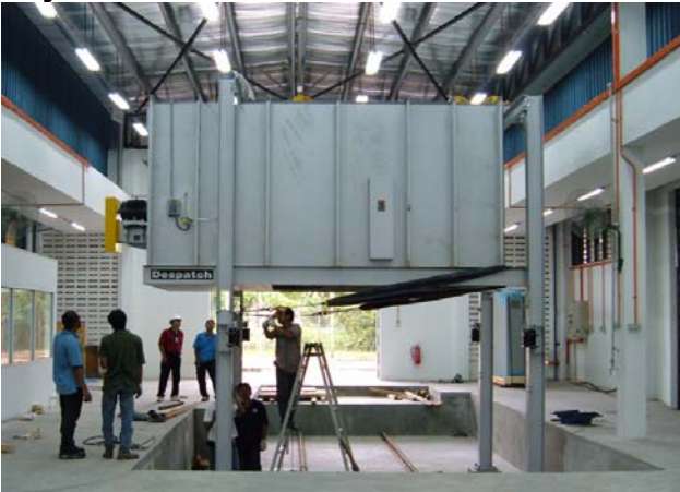
Figure 2: The furnace body is raised and secured between the four furnace columns.
