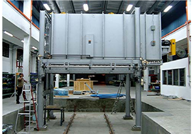
Figure 3: Doors hoisted and air plumbing completed. The very tight space for using lifting equipment and the pit made any placement of the heavy pieces a challenge.
