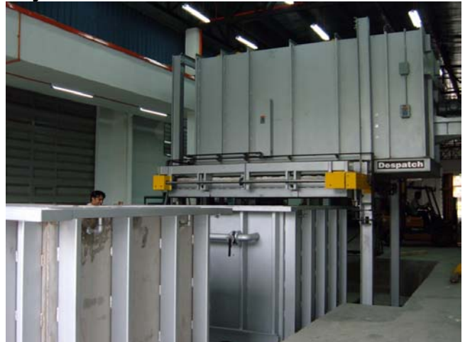
Figure 4: All major components installed and connected. (Furnace, Mobile Quench Tank and stationary rinse tank)
