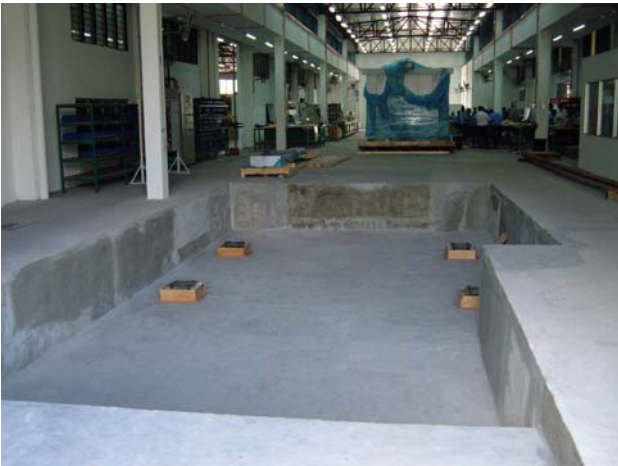
Figure 1: The start of the project. A concrete foundation consisting of a shallow pit is a part of the installation. The foundation was completed prior to the start of installation.
