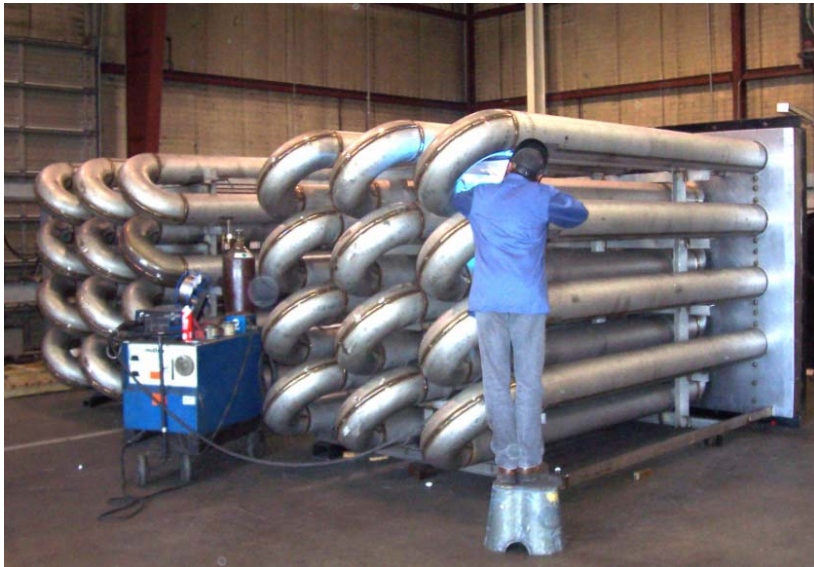
The picture show the two burner plugs getting the last welding performed during fabrication.
